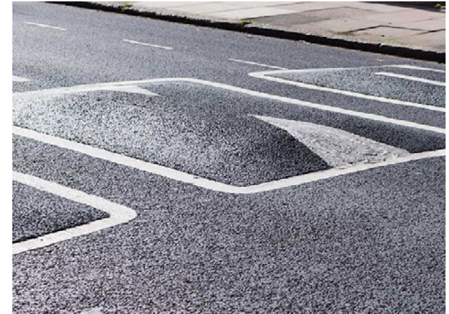
Figure 59: Example of a speed cushion.
