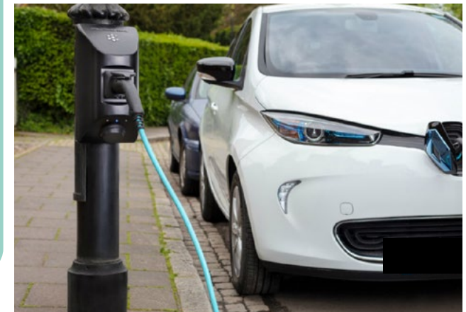
Figure 74: Example of on-street electric vehicle charging points.
