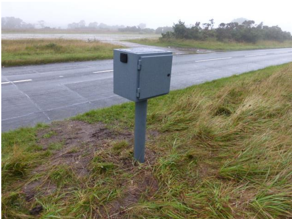
Figure 20: ATC Control Box and Loop
