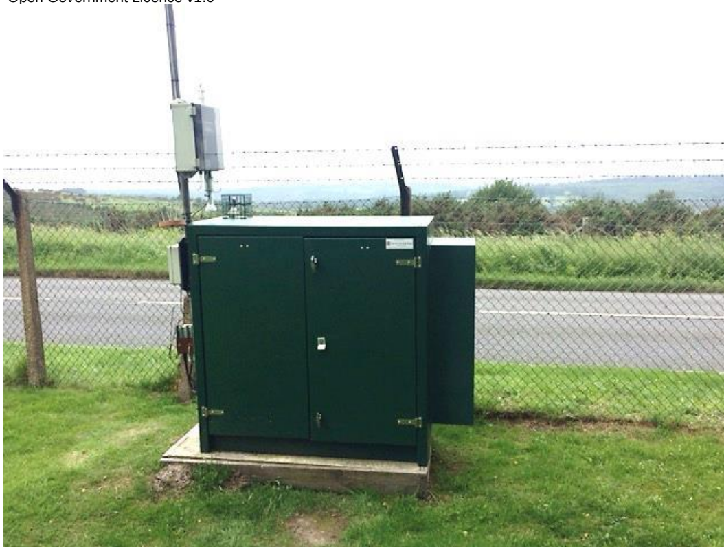
Figure 3: Automatic Monitor Enclosure at Kingstanding Police Training Grounds
