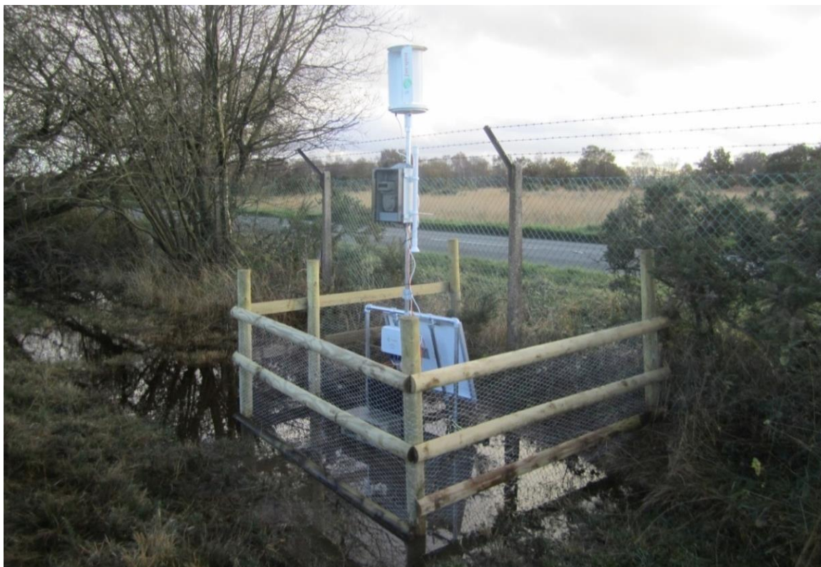
Figure 16: DELTA Sampler, Wind Generator, Gas Meter, Solar Panel (and Moat) (Site D4)
