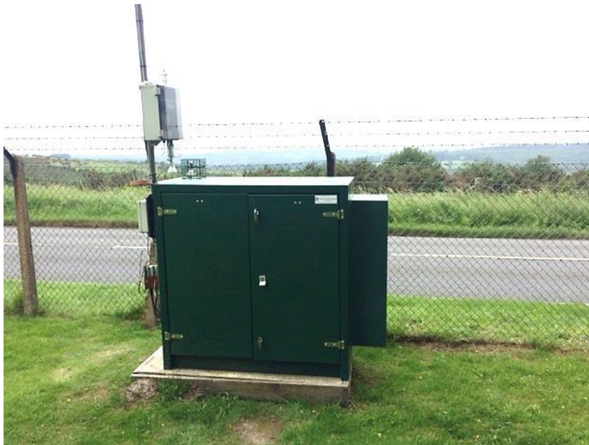
Figure 4.1: Automatic Monitor Enclosure at Kingstanding
