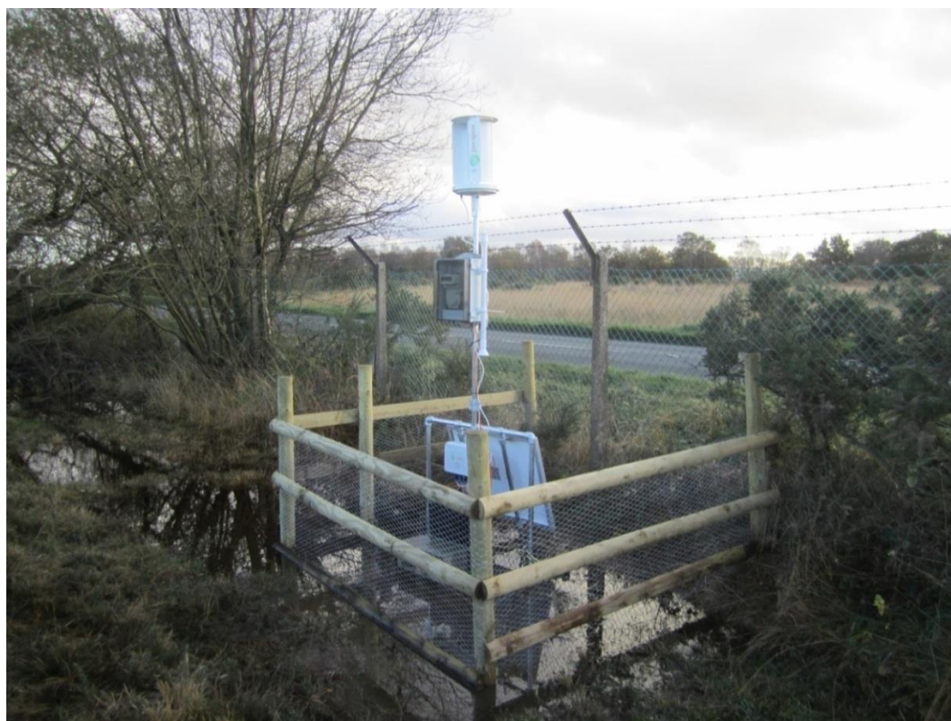
Figure 4.3: DELTA Sampler, Wind Generator, Gas Meter, and Solar Panel (Site T71)
