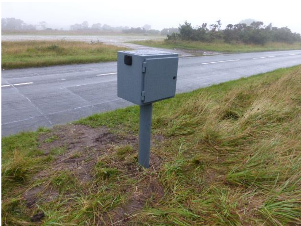
Figure 4.7: ATC Control Box and Loop
