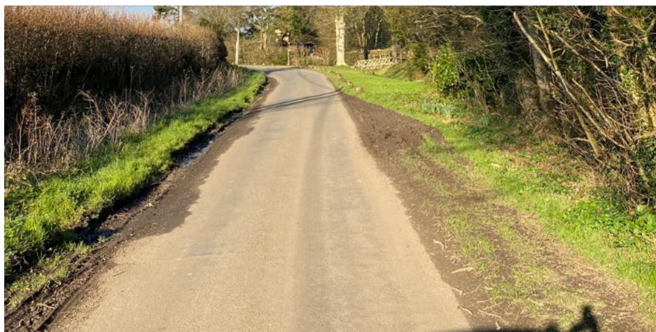
Examples of Damage to Verges
