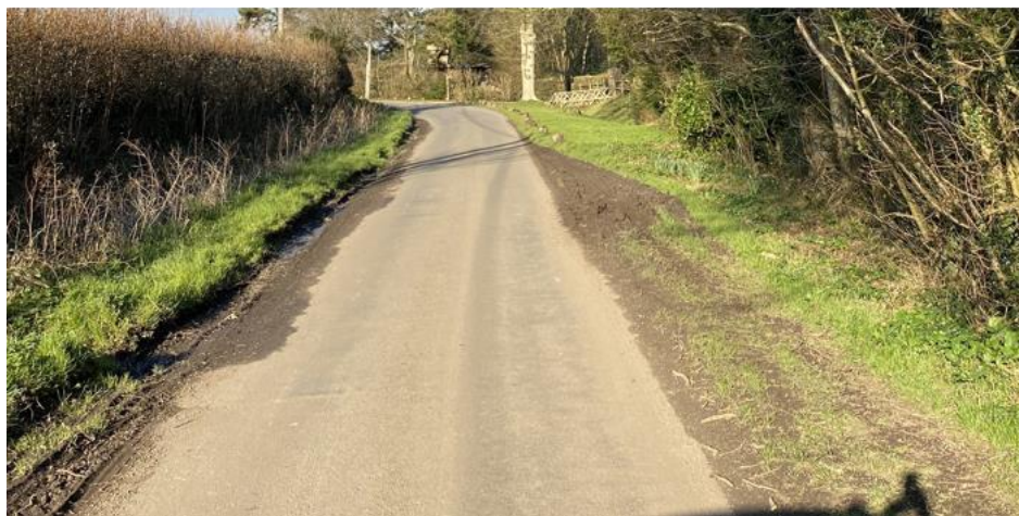
Examples of Damage to Verges
