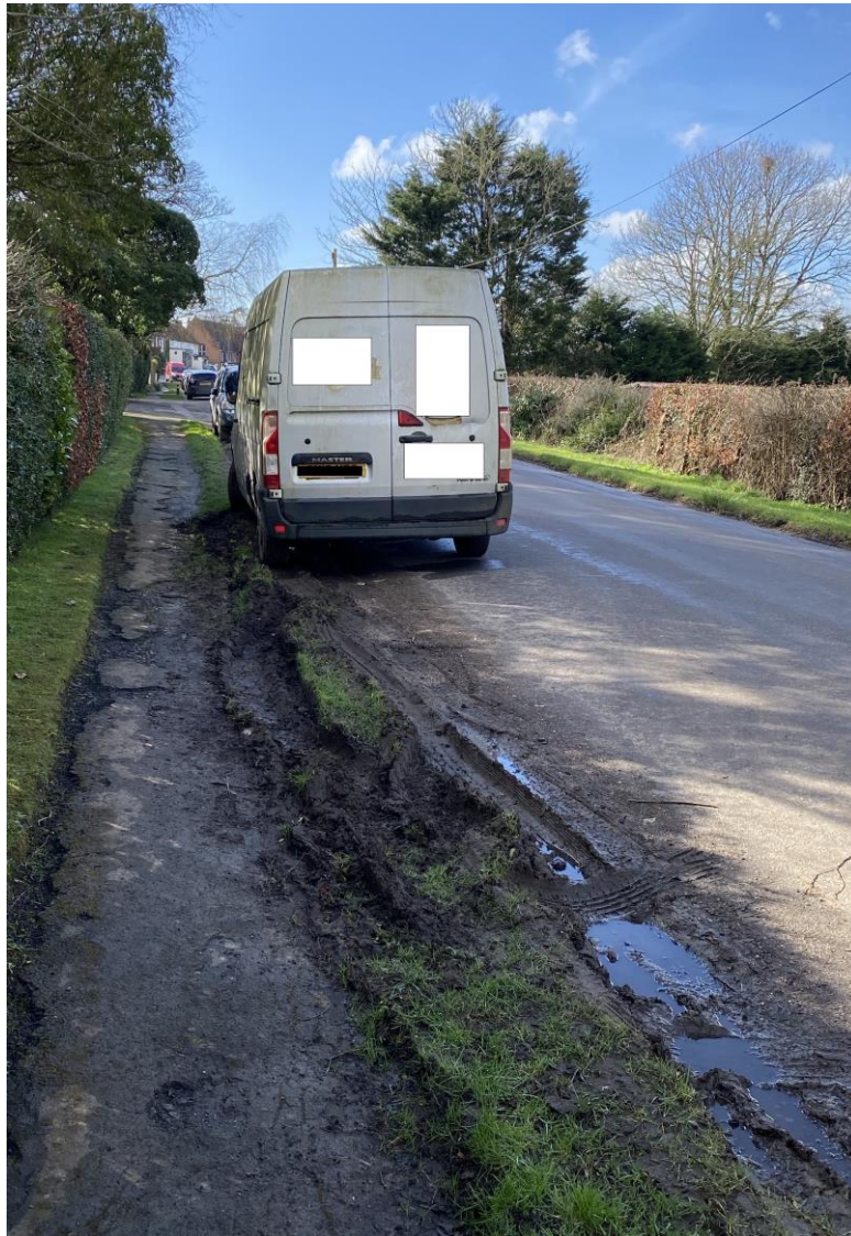
Damage to Verges on Waldron Road
