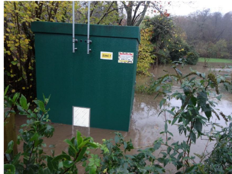
Photograph 8 – Flooding at Stream Farm
