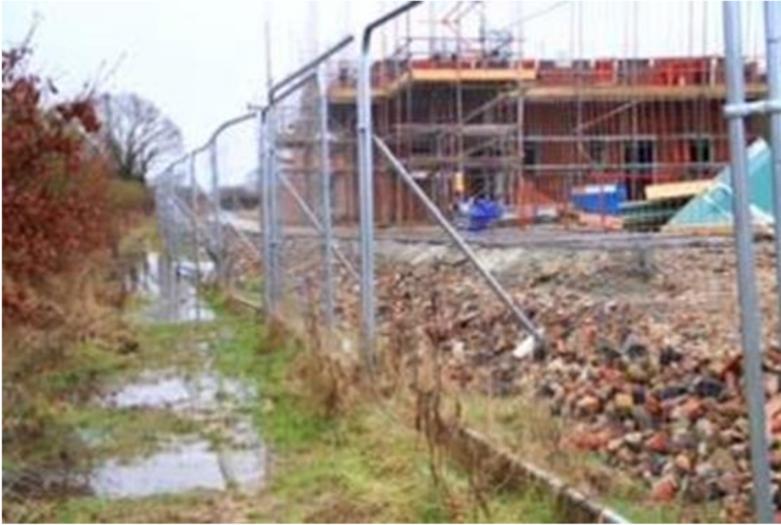
Feb 2017 – Bovis Homes Site – High Finished Ground Level and Water Run-off Pooling Adjacent. Photograph provided by D Phillips.
