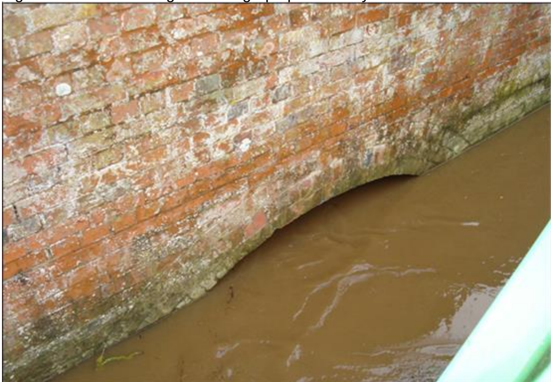
Nov 2016 – Water Level passing under A271 after one night of rain – Storm Angus. Photograph provided by N Downes.
