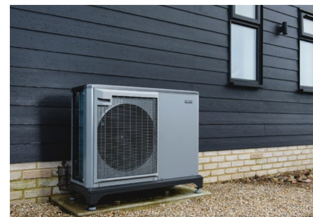
Figure 137: Example of an electric heat pump that is placed to the back of the house, whilst its grey colour fits nicely with the black weatherboarding of the property.
