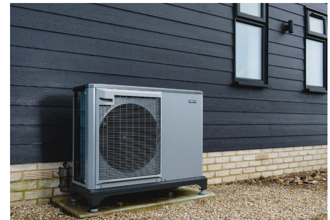
Figure 137: Example of an electric heat pump that is placed to the back of the house, whilst its grey colour fits nicely with the black weatherboarding of the property.
