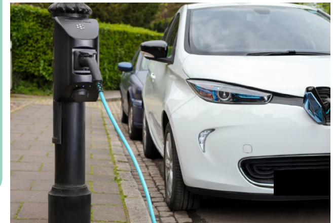
Figure 74: Example of on-street electric vehicle charging points.
