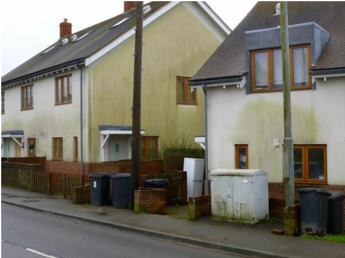
Detail of degraded rendering and services equipment impacting on frontage outlook. Also, lack of suitable provision for bins.
