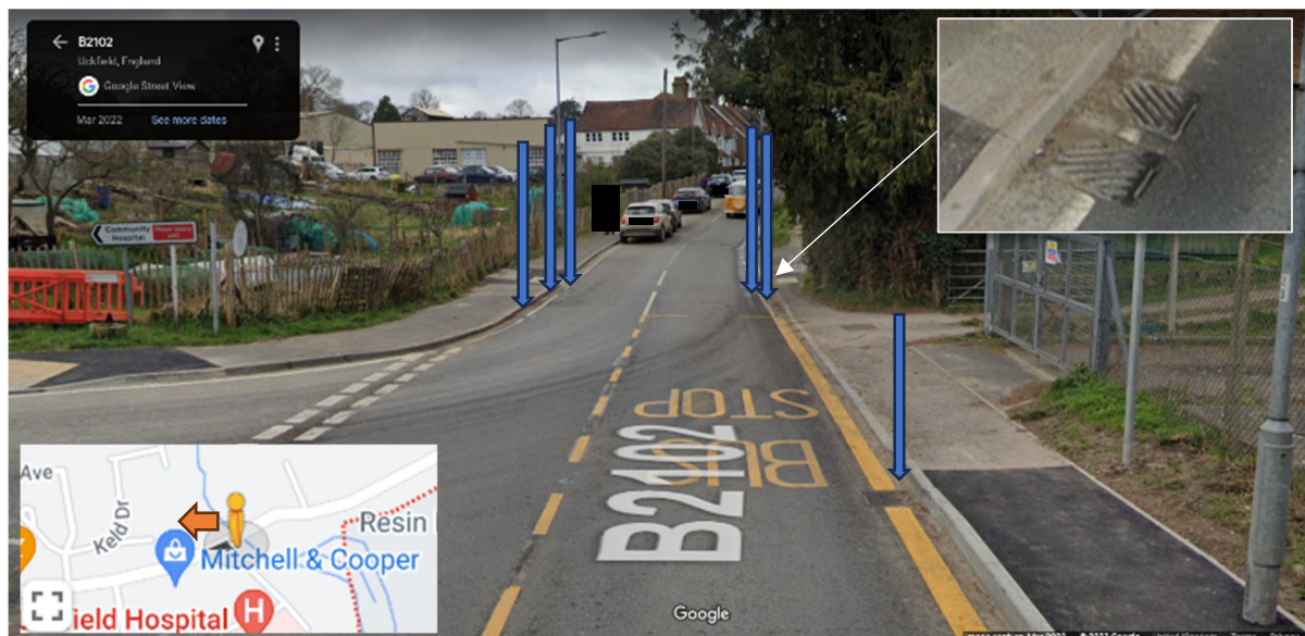
Figure 11 - Google Street View images showing location of the road drainage gullies, inset image showing double gullies blocked with sediment, which is likely to be a frequent occurrence (Imagery ©2023 Google).
